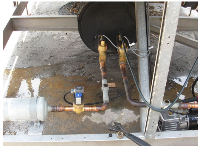
Upgrades to EXVs
